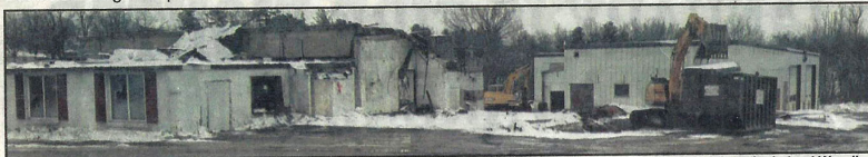
The outer shell of the old plant is lowered to one level.
