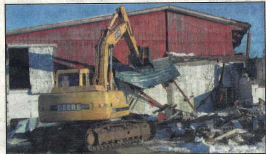
There were large chunks of metal in the debris.
