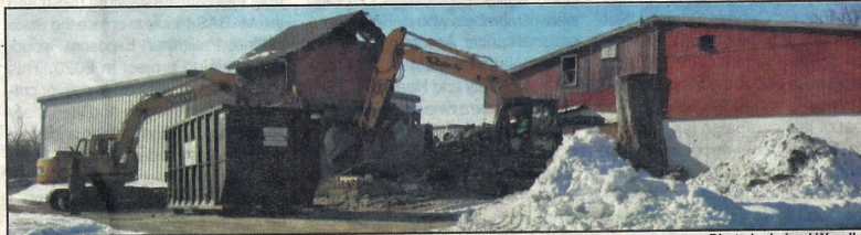
The front end loaders hoist the second floor of the house into a dumpster.
